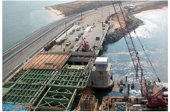
Wantagh bascular span drawbridge over sloop channel - Completed 2010. First brand new from the ground up bascular span drawbridge completed on Long Island in past 40 years. This electrical project included complete electrical and control systems, submarine cables, bridge operation, generator building, lighting, etc. Just to the left of this bridge is the temporary by-pass bridge completed electrically by Hinck Electric in 2001.
