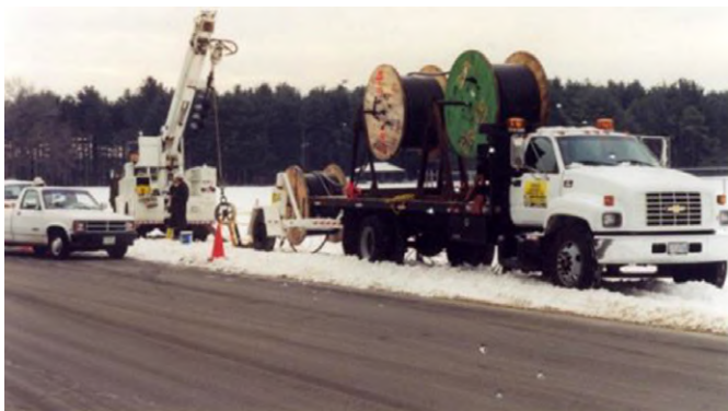
Installation of 15KV 750MCM cable at Brookhaven National Laboratory. Part of Hinck's highly acclaimed, three year upgrade project at BNL which included four brand new 13.8KV to 2.4KV substations, new 13.8KV and 2.4KV feeders, new duct banks, and related high voltage splicing and terminations.
